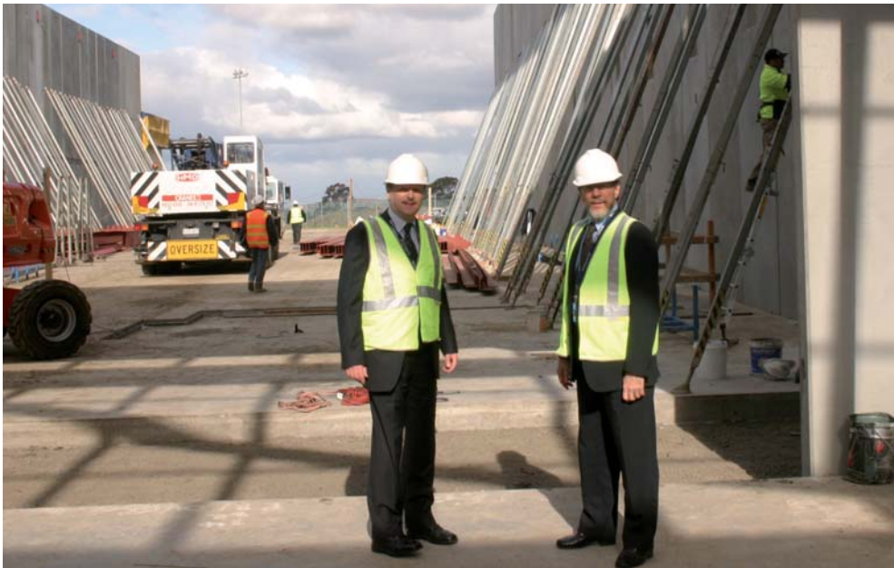
Graeme Thompson, Chairman, right, and Myles Curtis, Managing Director, left, assess progress during construction of Security's plant expansion.
