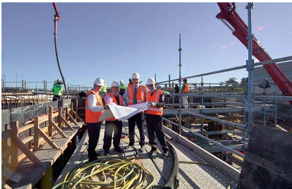
Frank Campbell, Assistant Governor (Corporate Services), second from left, discusses progress on construction of the business resumption site with, from left to right, Greg Graham, Richard Mayes and John Wightman, members of the Reserve Bank's project team.
