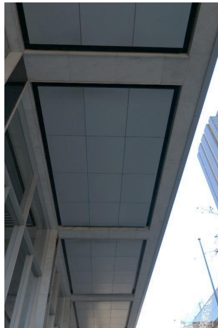
Figure 13 – General view of the podium soffit adjacent to the north side of the RBA Head Office entry. Note the original suspended marble soffit was replaced in c2001.
