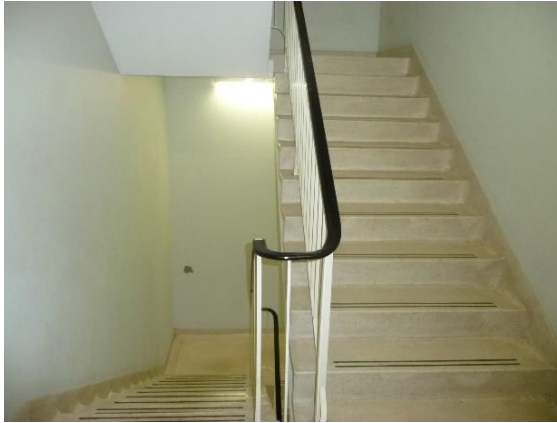
Figure 16 – Example of fire stair finishes and painted steel balustrades within the RBA Head office building.
