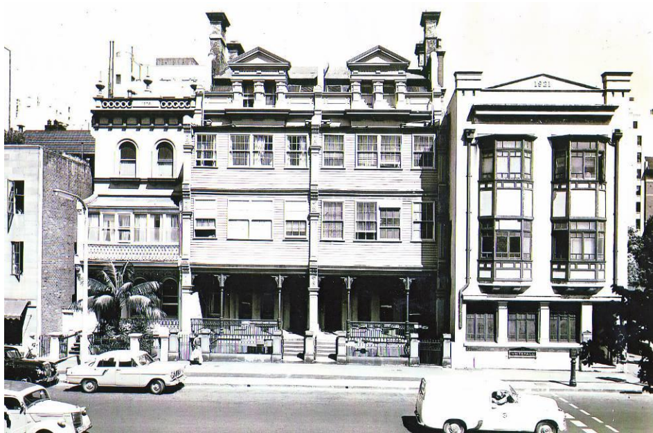
Figure 52 – View of the houses located at 219-215 Macquarie Street Sydney, which were demolished for the construction of the Reserve Bank in 1959.
