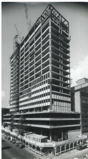
Figure 6 -View of the northwest corner of the RBA Head Office showing the original marble panels being installed to the north and west elevations, c1962. Source: National Archives of Australia.
