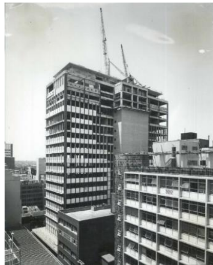
Figure 5 - View of the south and west elevations during construction c1962. Source: National Archives of Australia
