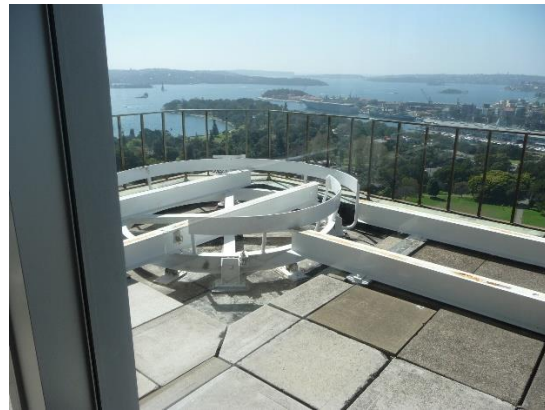
Figure 29 - General view showing the concrete pavers and access equipment for servicing the exterior of the RBA building.
